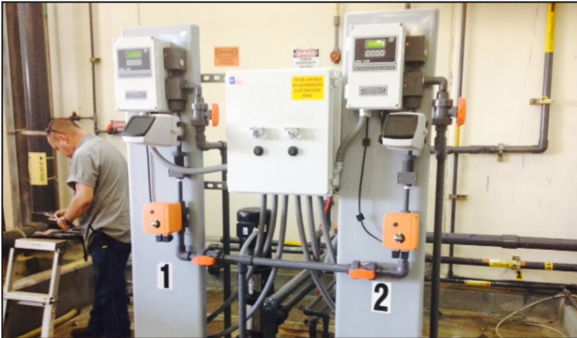
Replacement of bleach pump with special vacuum feeders eliminated frequent pipe and valve leaks that were caused by running the pump at 100% capacity just to get close to what was needed.
