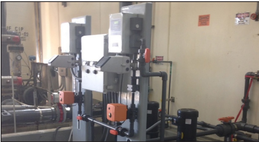
Replacement feeders gave operators new capability for providing required bleach dosage, and also for controlling it from the plant's SCADA terminal.
