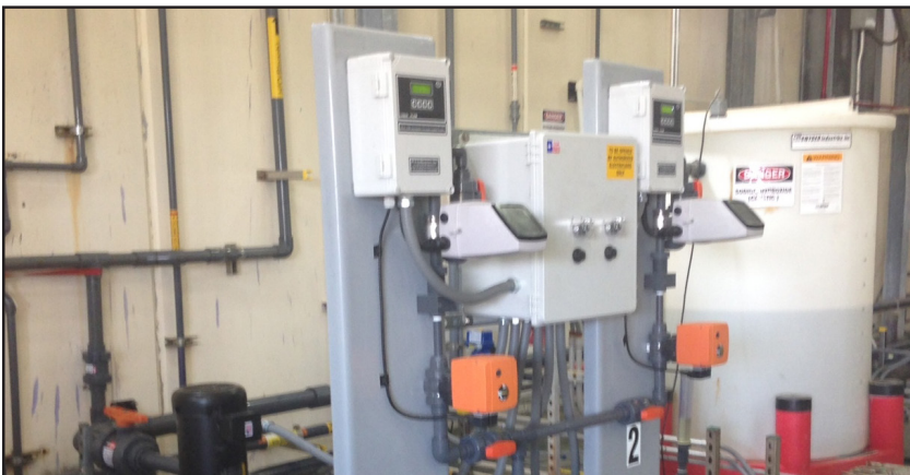
Replacement feeders require much smaller footprint than was previously needed for bleach delivery mechanism, and their installation has also resulted in greatly reduced CIP frequency.
