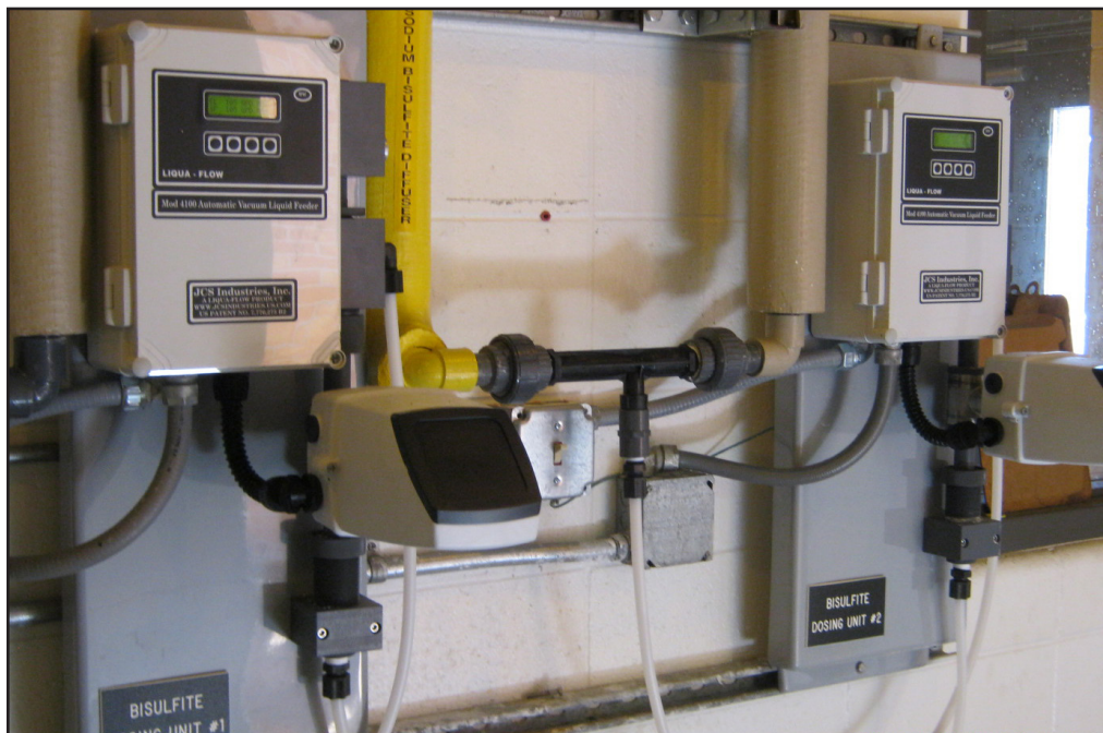
Replacement liquid vacuum bisulfite feeders provide more reliable dechlorination for zero discharge to effluent, while enhanced control lowered bisulfite usage by 30%.
