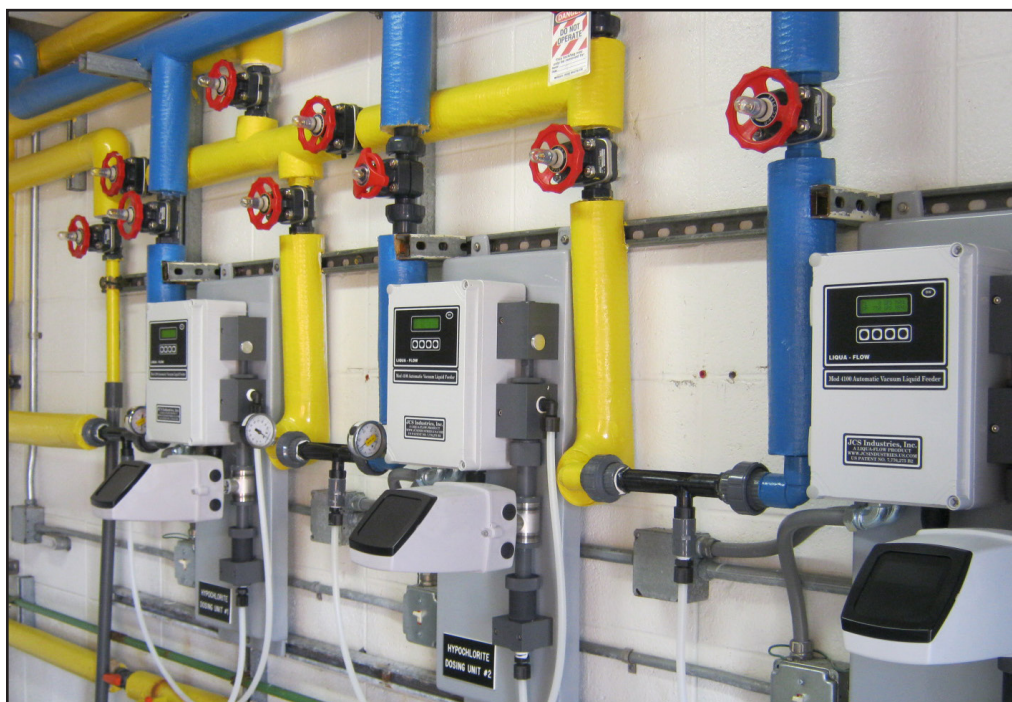
Replacement liquid vacuum hypo feeders provide more reliable chlorination for disinfection requirements.
