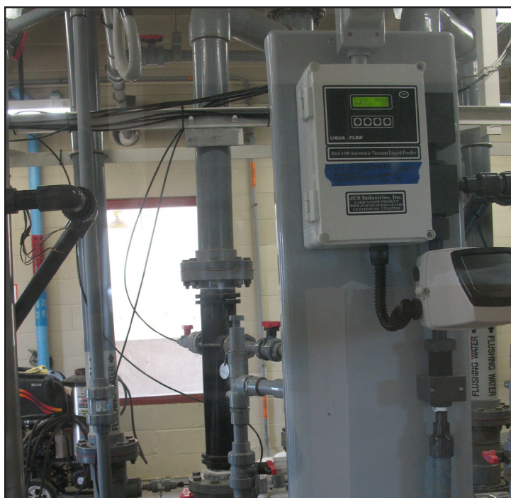
Since replacement vendor was able to match exact same previous feeding configuration, installation consisted of fitting the replacement units on the same platform, using the same conduit, and making adjustments to the PVC piping for the inlet and outlet.
