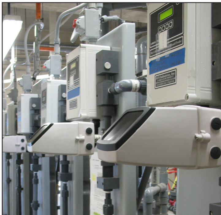
Each of seven replacement units feeds hypo at approximately 800 gpd, into a group of three contact chambers that hold total plant effluent pending discharge. Capacity of each hypo feeder is 10,000 gpd. Major plant revisions are in construction.
