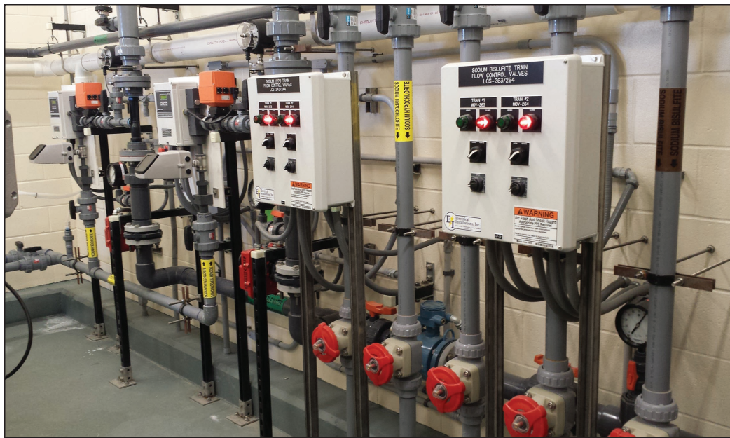
Similar feeder system is also used to deliver sodium bisulfite (NaHSO 3 ) to provide for dechlorination of CSO discharge.
