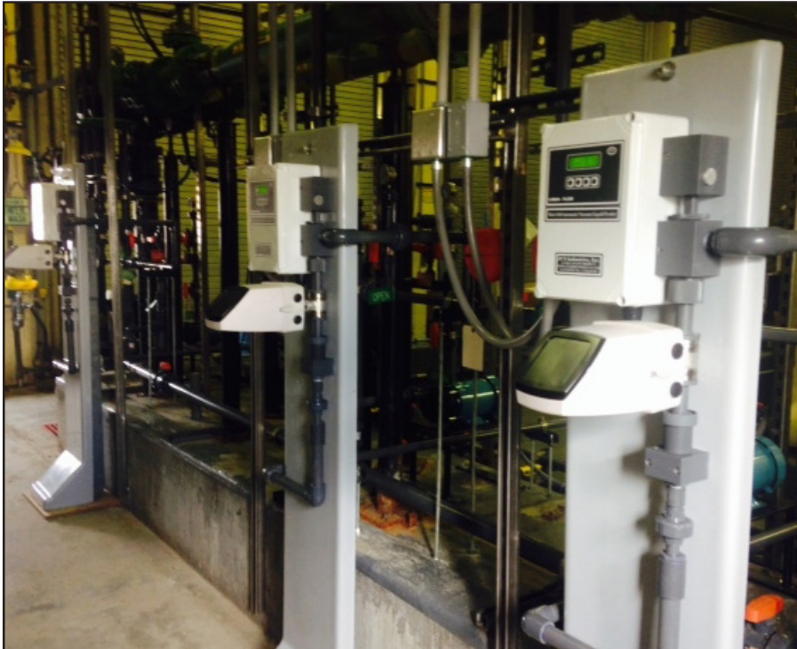
At the city's 1200 MGD WTP, 15% hypo is fed at the main entry point to distribution shafts, at the rate of 1000-1200 GPD.
