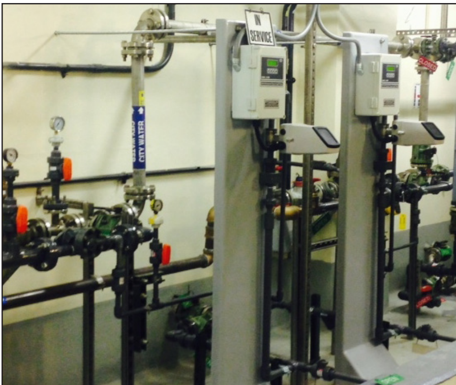
At the city's 80 MGD WTP, 15% hypo is fed at the rate of 120-150 GPD.
