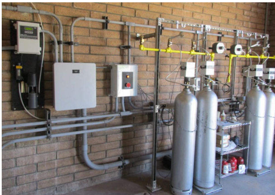
Special gas chlorination system significantly enhanced safety for gas option for disinfection, while offering other unique components and controls for reliability and efficiency.
