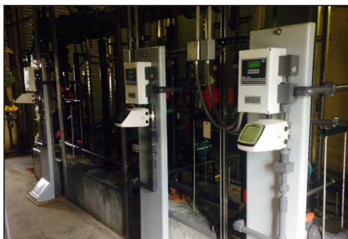
For the city’s original use of the advanced vacuum feeder units for hypo feed, now in sixth year at both 80 MGD and 1200 MGD WTP’s, the need was to improve reliability and reduce maintenance for less advanced vacuum feeders. Those less advanced vacuum feeders had been installed years earlier, also to improve reliability and reduce maintenance vs. metering pumps.
